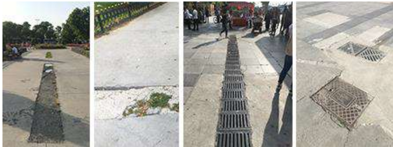
Fig. 14. Problematics on floor covering in Kadıköy Square (Source: Kutsal Göllü, Canbay Türkyılmaz, 2018)
