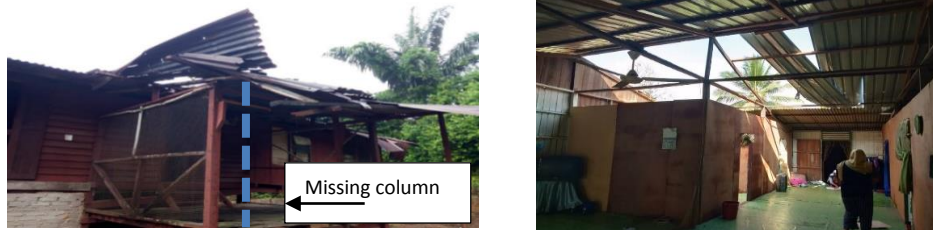
Fig. 3. (a) Loss of vertical column support and overhang roof damage; Post Restricted Use with barricade the front portion (b) Purlin and rafter section sizes were inadequate and purlin-rafter connection failure and roof blown away) Damaged interior contents due to broken fallen roof sheathings; rain water intrusion; Post Unsafe with falling hazard
