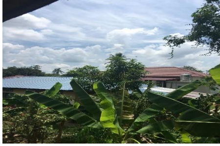
Fig. 8. (a) Adjacent rural homes with newly built roof with thicker roof sheathings did not experience any damage (b) Wind damage to interior walls and possibilities of damage to vertical support structural system when the roof was breached
