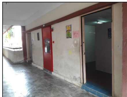
Fig 1. The condition of toilet in AB
