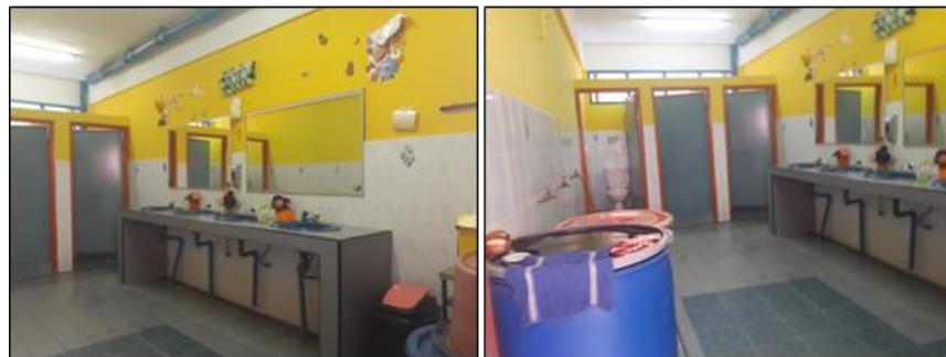
Fig 2. The condition of toilet in BC
