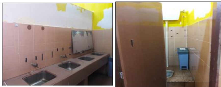
Fig 3. The condition of toilet in DC
