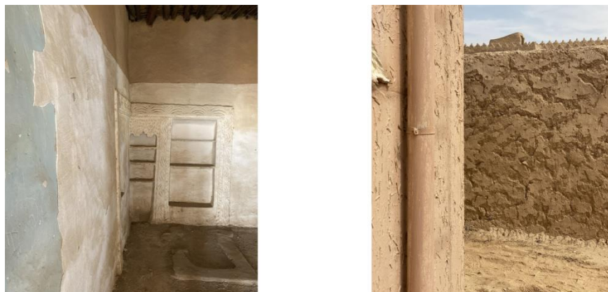
Photo 4.4& 4.5 lousy conditions of the mud walls (Source: author)
